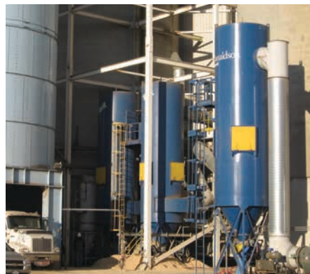
RF - Grain Terminal 34,000 cfm (57,754 m 3 /h)
