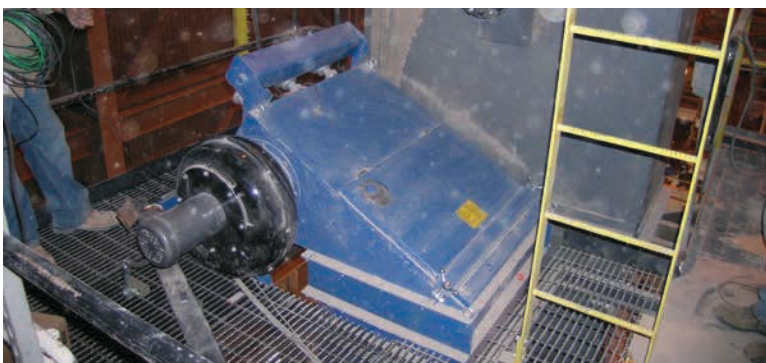
CPV - Bucket Elevator 1,200 cfm (2,038 m 3 /h)
