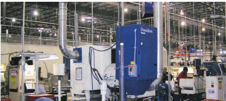
WSO at M3 Achining Center 1,200 cfm (2,038 m 3 /h)
