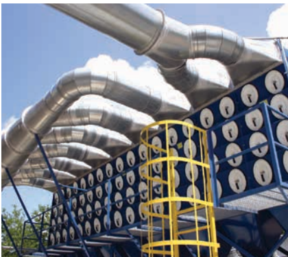
DFO on Sawdust 57,500 cfm (97,692 m 3 /h)
