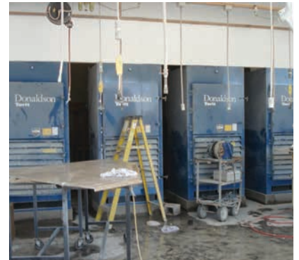
DWS on Granite Finishing 22,000 cfm (37,370 m 3 /h)
